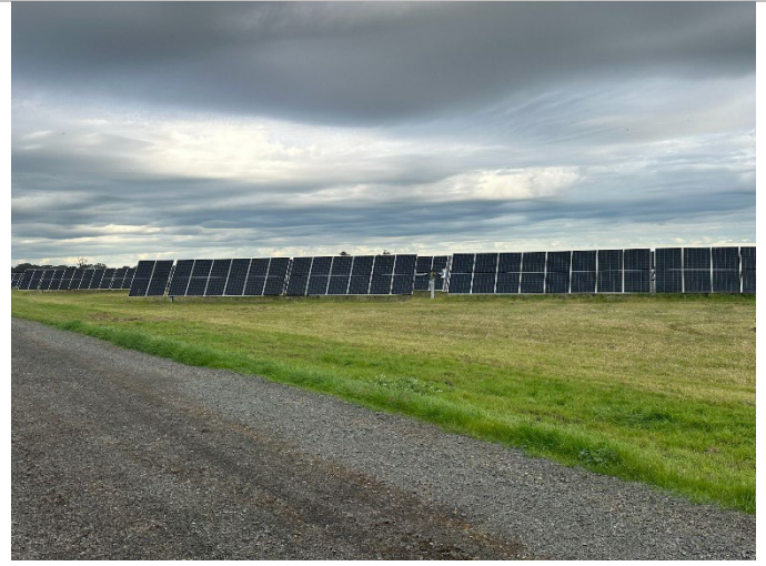
Photo 2: Solar panels and sealed internal access road
