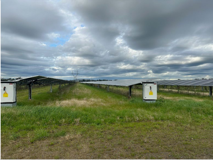
Photo 12: Solar arrays and inverters
