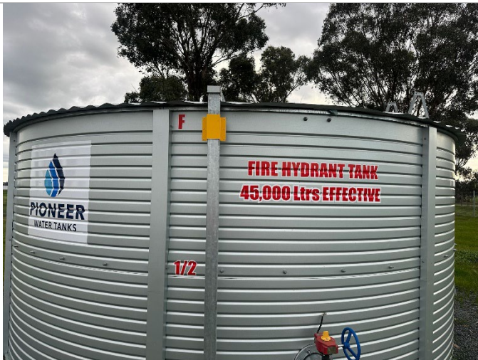
Photo 5: Fire water tank
