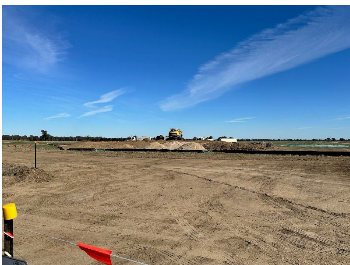
Photo 17: Stockpiled materials and sediment controls
