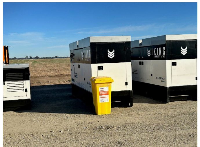
Photo 6: Spill kit and self-bunded generators
